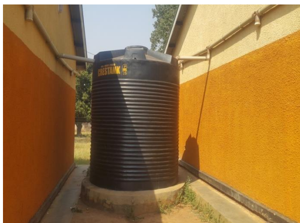
Figure 39: Water tank for rain water harvesting
