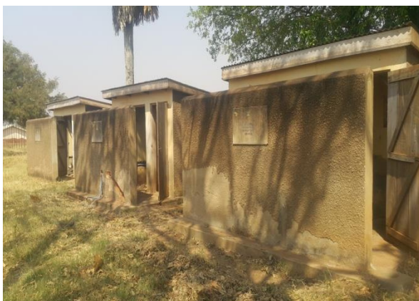
Figure 46: Old sanitary facilities
