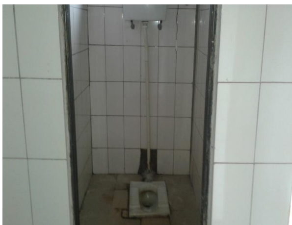
Figure 21: Sanitary facilities at the girls' dormitory
