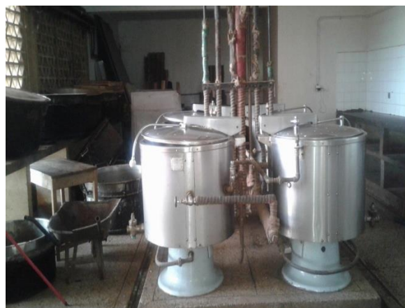
Figure 39: Boilers in the kitchen
